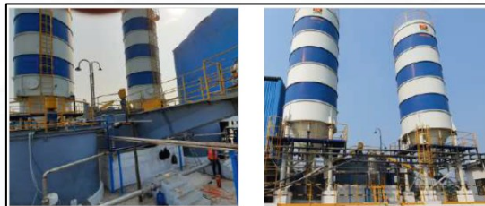
Slurry Preparation Plant - Gujarat
